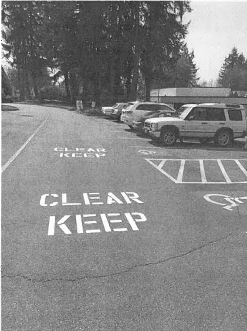
Please keep the space that says "Keep Clear" open at all times.
